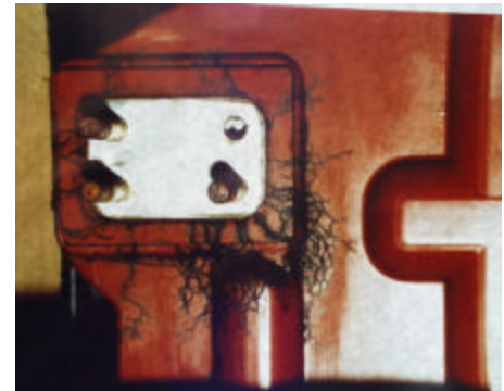
This dangerous tracking was located deep within the switchgear.
