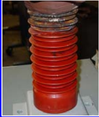
Active Partial Discharge & tracking found; before failure occurred!
