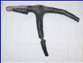
Bad cable found before it failed!
